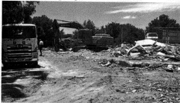
The first stage of the redevelopment of Stirling's old Shell petrol station is underway, with the structure now entirely demolished. Developer Frank Agostino plans to build an Agostino Always AM/PM service station at the site on Merrion Terrace. However final plans for its redevelopment are still pending full approval from the Adelaide Hills Council. The council said they had received a number of enquiries about the redevelopment of the site and complaints about its appearance while undeveloped.
