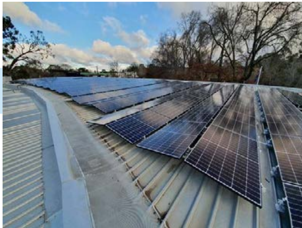
Solar panels on the roof of Coventry Library, Stirling.
