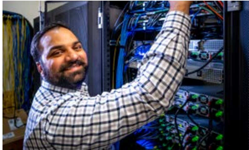
Senior ICT Officer, Yashmeet Sandhu, inspects Council's servers.
