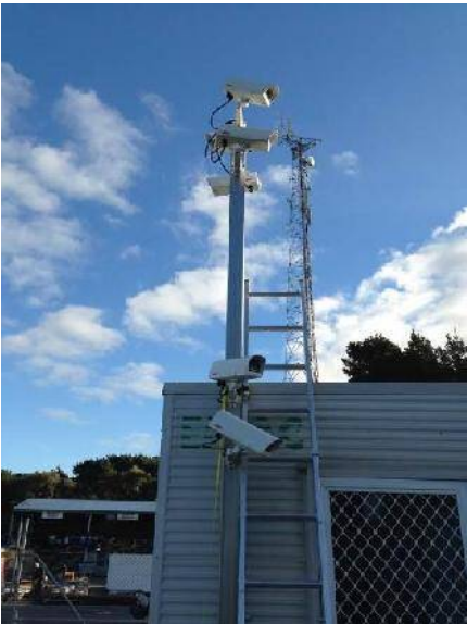
New Weighbridge Processing System installed at Windmill Hill Transfer
