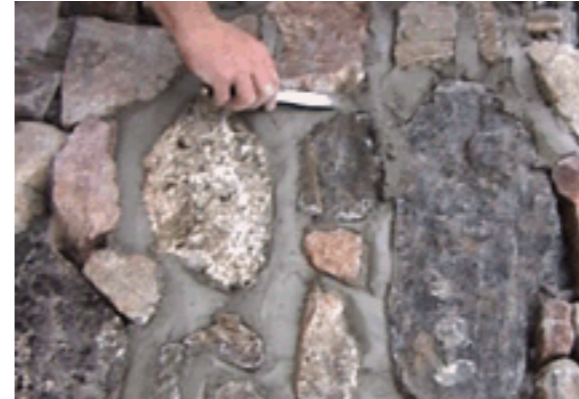
Opportunity for stone pitching in spoon drain to create rills and channels
