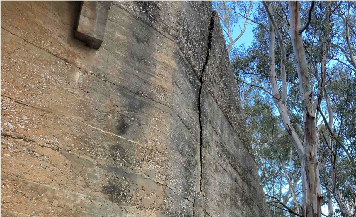
Figure 2-6. Burfords Hill Road bridge, south-west wingwall showing significant cracking
