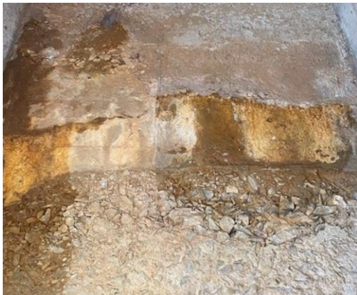
(a) Abutment concrete fretting
