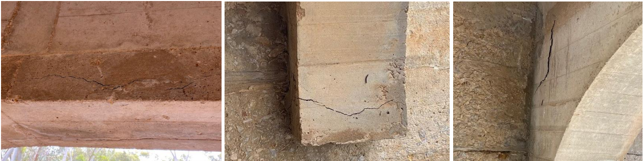
(a) Western girder soffit cracking
