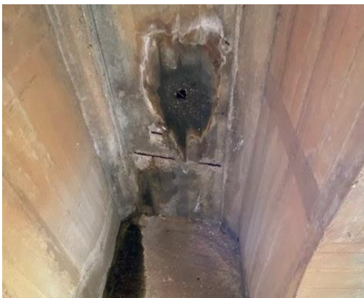
Figure 6 Concrete Surface Efflorescence and Water Stain
