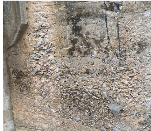
(b) Abutment and wingwall concrete fretting
