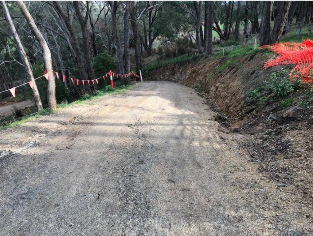
Looking down the new property access, with the encroachment on the right.
