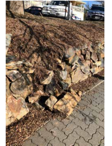
Maintenance issues to be addressed.
