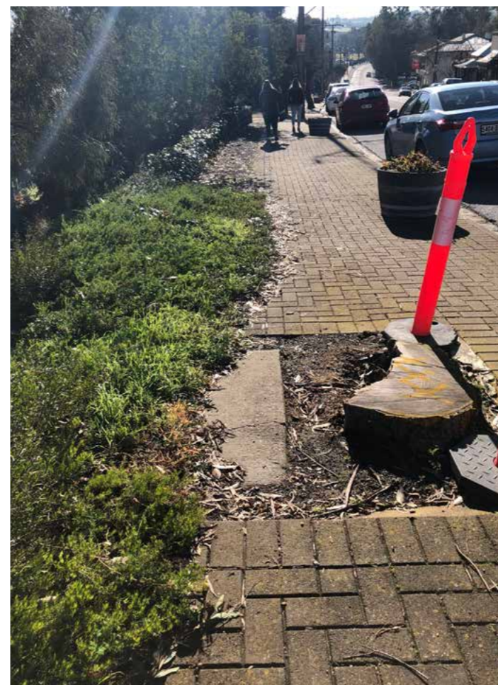
Historical pruning regimes due to the power lines have affected street tree health.
