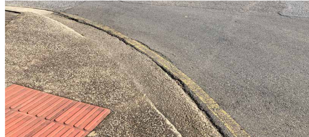
Pram ramps for crossing, a wide road and vehicle speeds are issues outside the Gumeracha Hotel + Albert Street generally.
