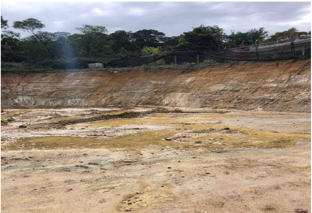
Photo 2: Site works for the foundations of the new supermarket building – view of northern eastern boundary
