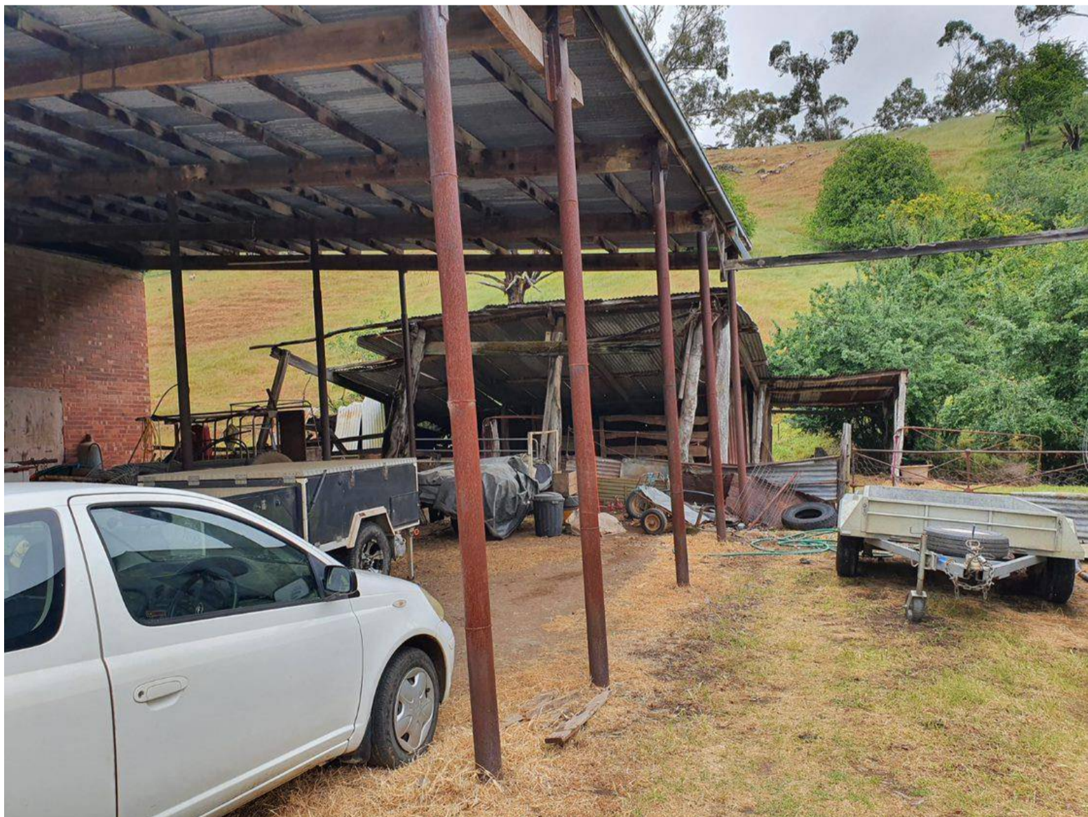
Description: View of dilapidates former milking shed
