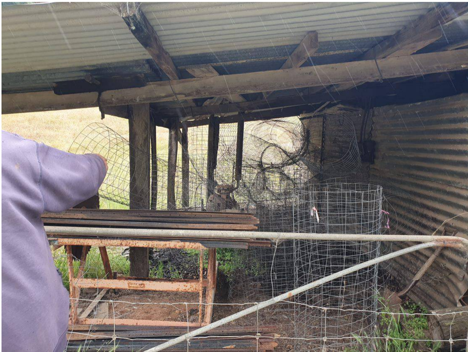
Description: View of pumping equipment in spray shed
