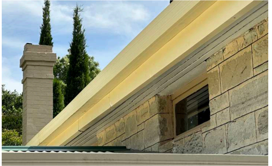
Figure 10 – Former Coach House, detail of later window and original chimney, West Elevation
