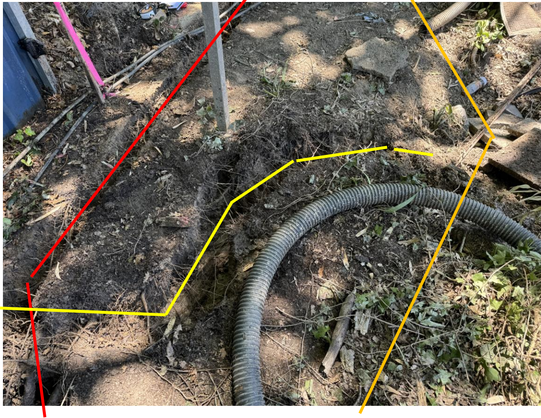
Red line shows the proposed retaining wall Yellow line the major root Orange line indicates the new location of the retaining wall
